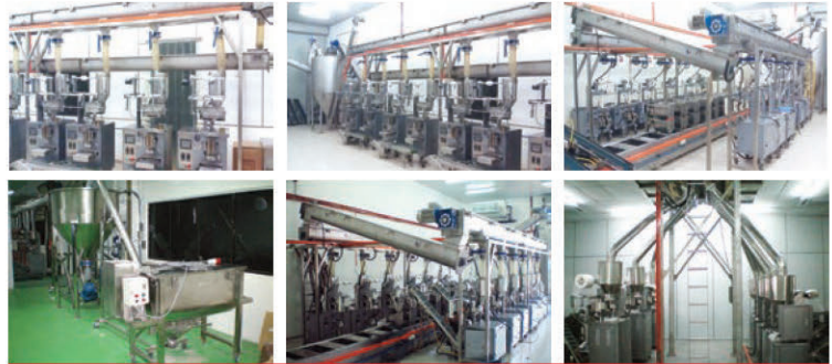
Automatic Powder Mixing & Handling System
